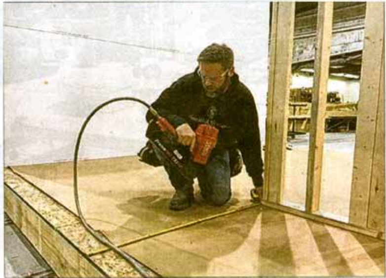
Tim Scarpelli, a framer at Unibilt, measures as he sets a wall on what will be someone's new home.
